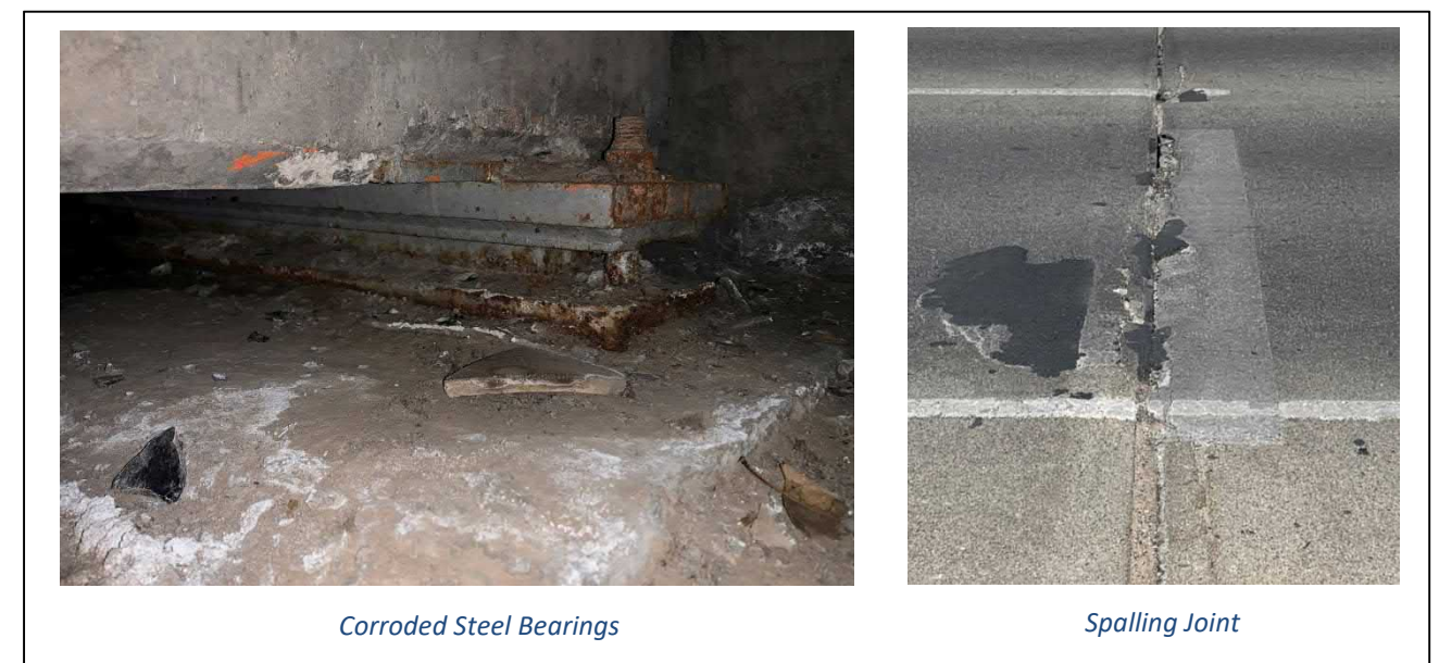
Exhibit 3-5, Existing Deficiencies of Bridge No. 6224
