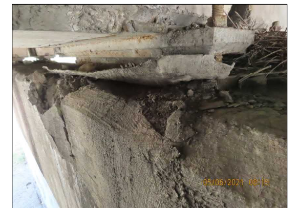
Delamination below one of the girder bearings of the eastbound bridge (photo courtesy of NMDOT)
