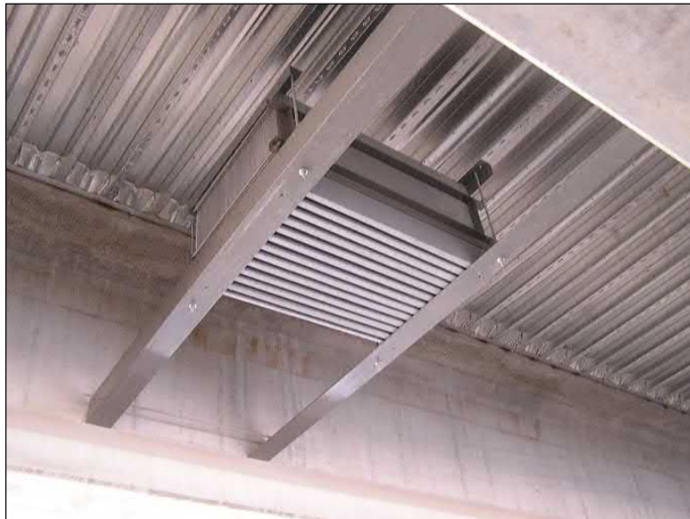
Exhibit 5-20, Example of a Bat Box Installed on a Recent NMDOT Project
