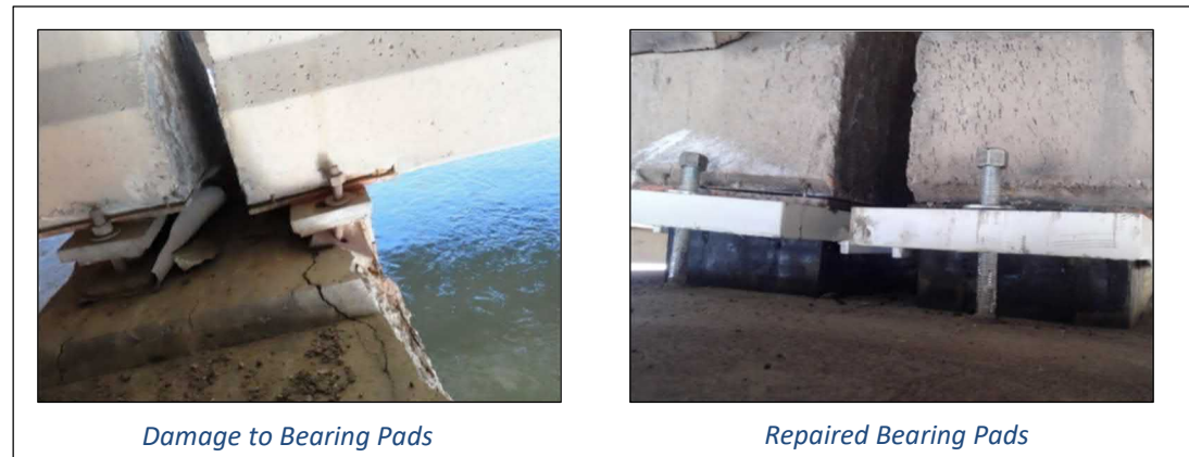
Exhibit 3-6, Emergency Repair at Pier 3 of Bridge No. 6224
