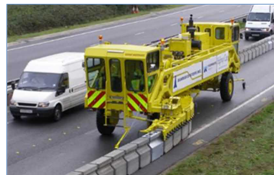
Road Zipper Movable Barrier System to provide a reversible lane during construction
